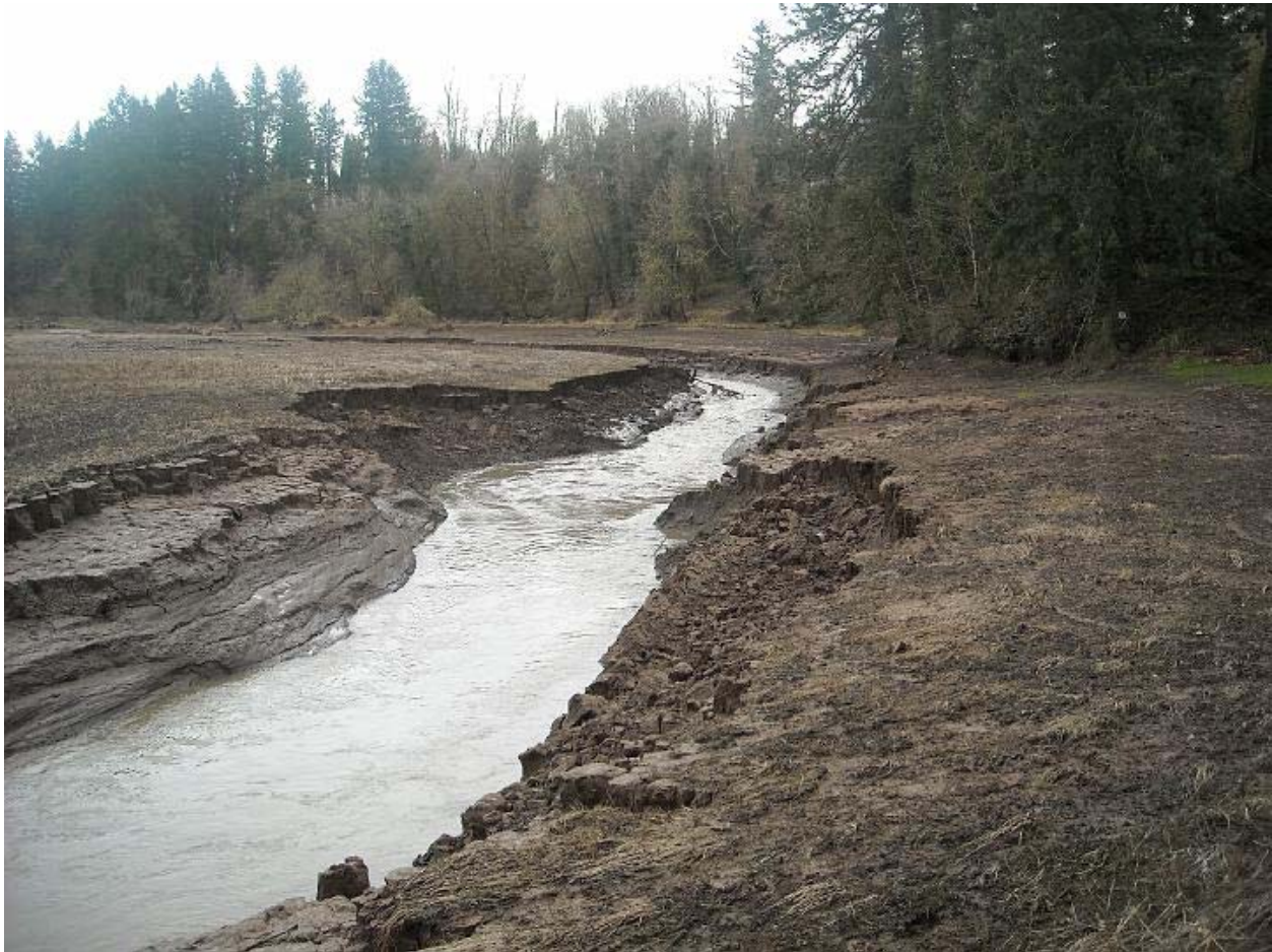
Figure 33. Sevvick Pond Sediments in the Channel Beaver Creek after the Dam Washed out in the January 2, 2009, Flood
